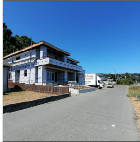
Photo 2: Looking northwest towards the new house and retaining walls from Battersea Road.
