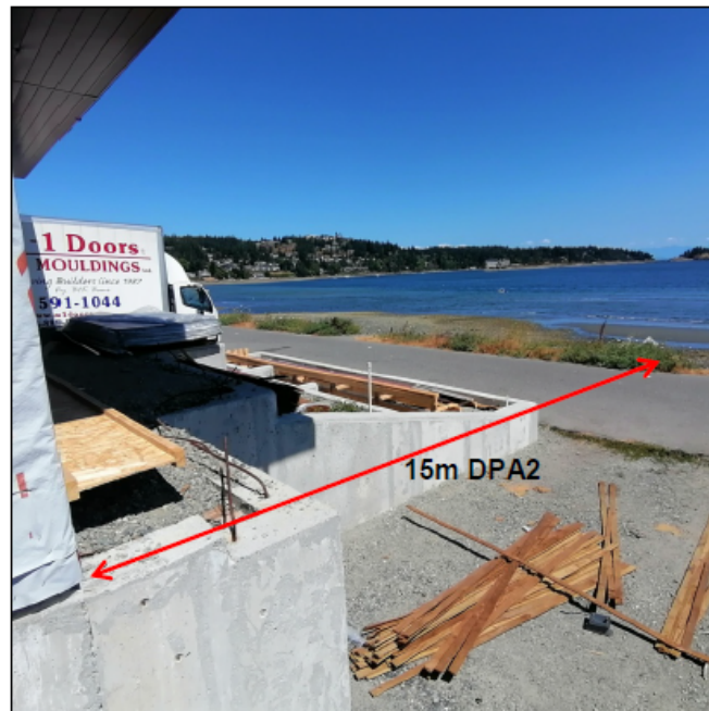
Photo 3: Looking northeast across Battersea Rd towards the ocean from the south side of the new house. The 15m DPA includes paved road, rip rap and the retaining walls. Photo 3b is looking across the concrete patio area under the cantilevered deck that has not been poured yet.
